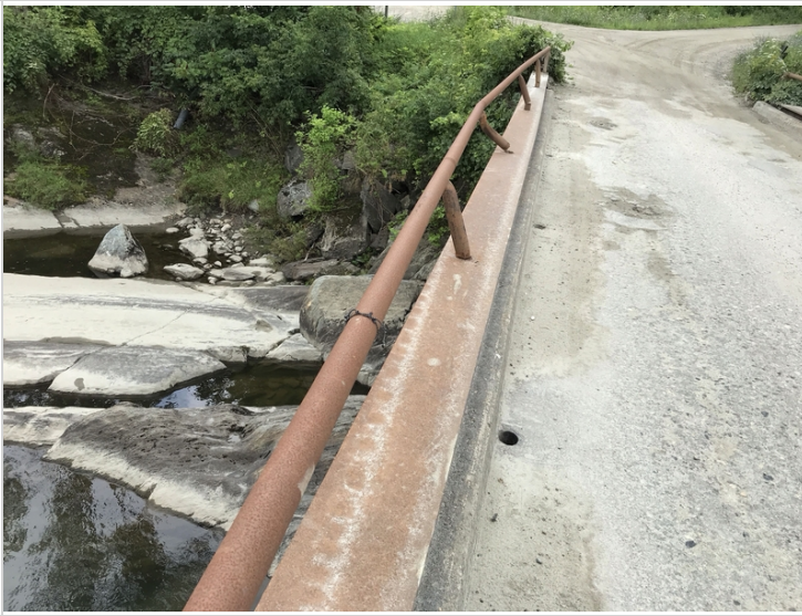
Upstream rail damage
