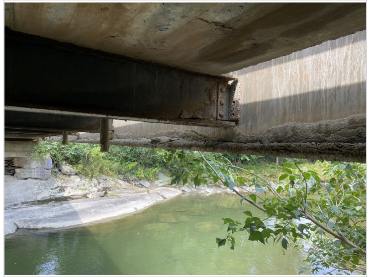
Beam #2 from Abutment #1 with Debris Build Up
