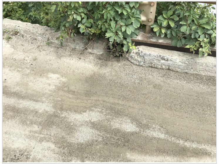
Downstream curb at abutment 2
