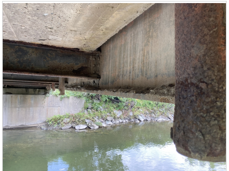
Beam #1 Lower Flange Build up of Material looking at Abutment #1
