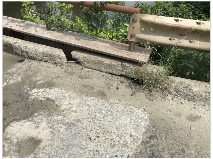
Downstream curb at abutment 1
