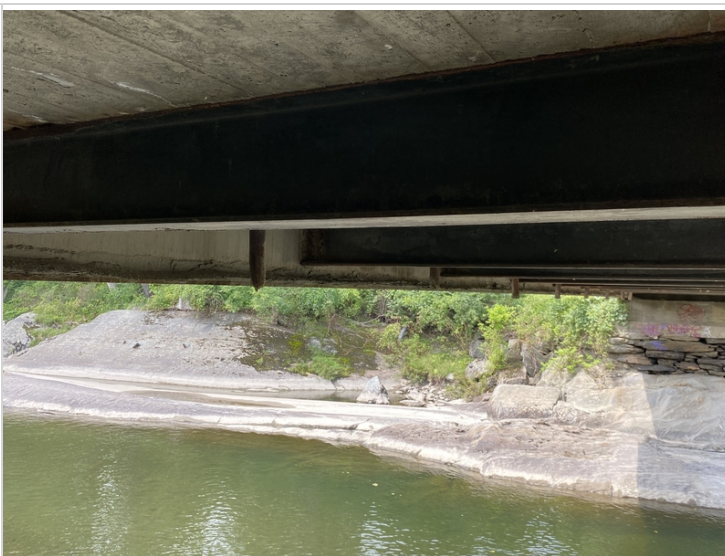
Beam #1 from Abutment #1 with Debris Build Up
