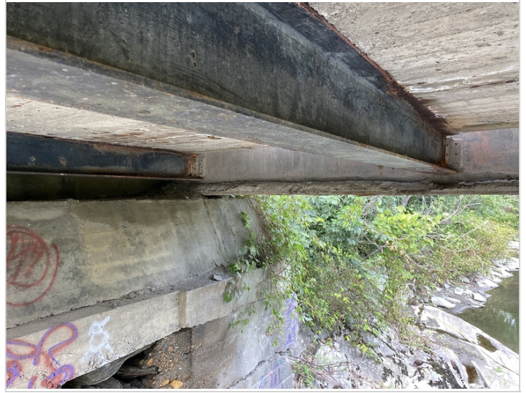
Beam #2 Lower Flange Build up of Material near Abutment #2
