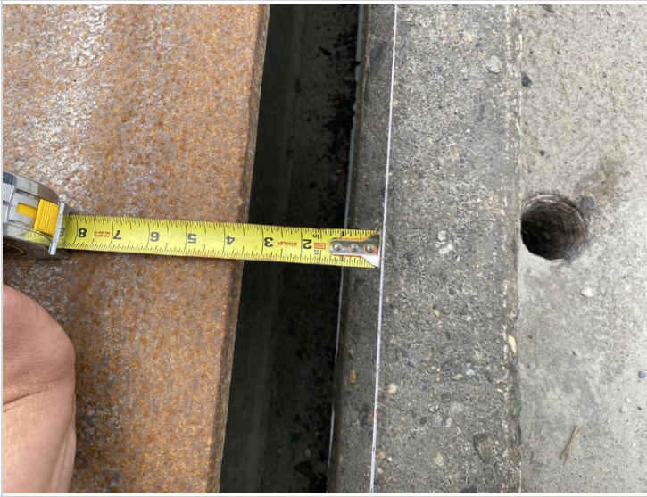
~3-3/4" of Downstream Sway in Downstream Beam #2
