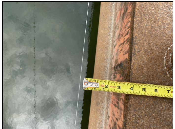
~3-3/4" of Downstream Sway in Upstream Beam #1
