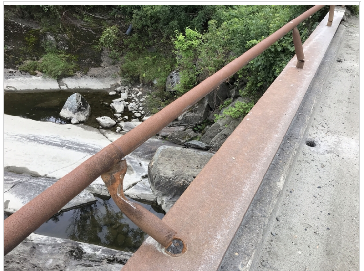
Upstream rail damage
