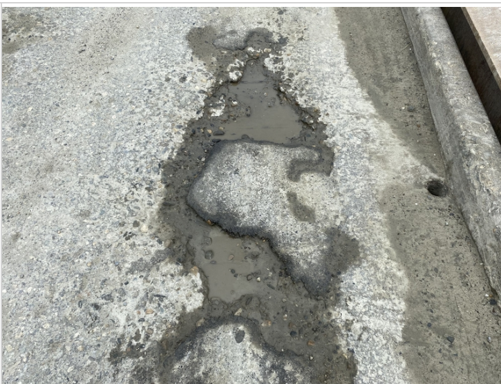
Spalling on Top Surface of Deck
