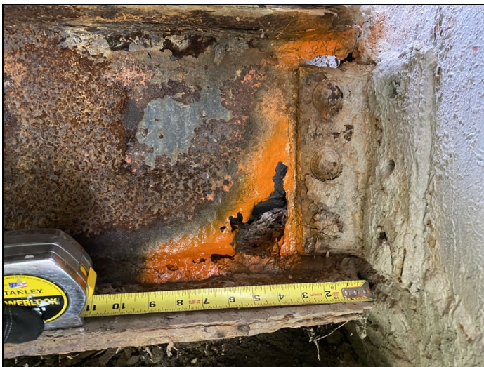
Floorbeam #0 Upstream Perforation
