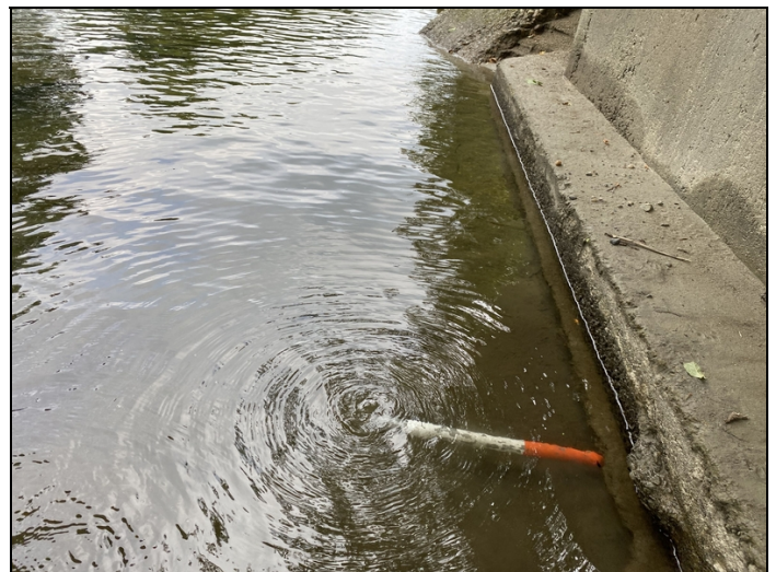
~2'-6" of Penetration below Abutment #1
