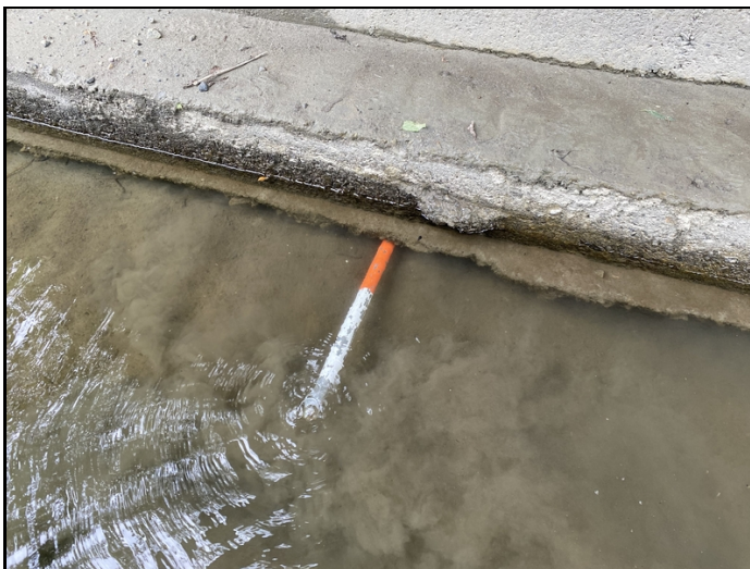
~2'-6" of Penetration below Abutment #1
