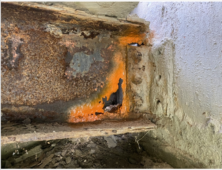
Floorbeam #0 Upstream Perforation
