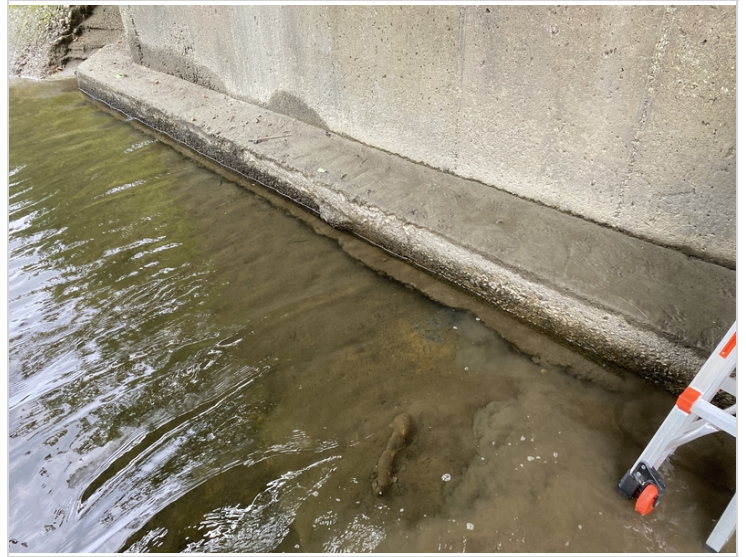
Abutment #1 Scouring / Undermining
