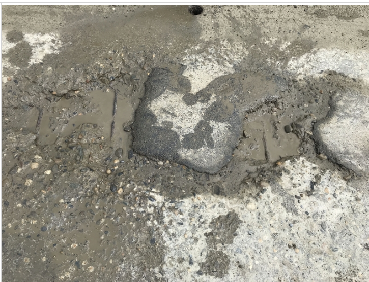
Exposed rebar in deck pot holes
