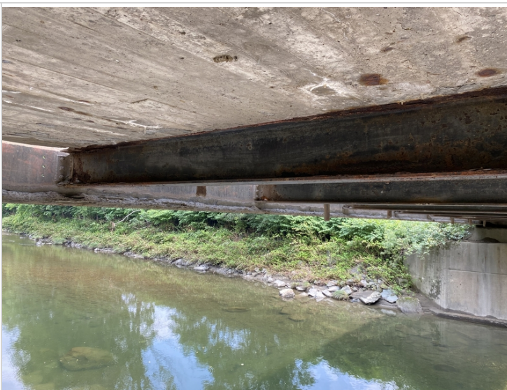
Beam #2 Lower Flange Build up of Material looking at Abutment #1
