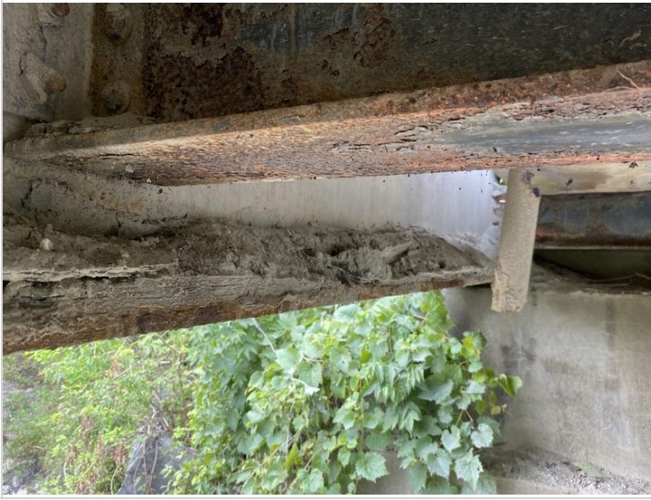
Beam #1 Lower Flange Build up of Material near Abutment #2
